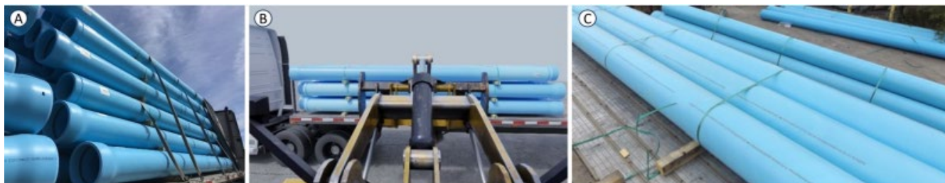
Figure 1. Pipe Bundles During Transport (A), Before Unloading (B), and After Incident (C)
